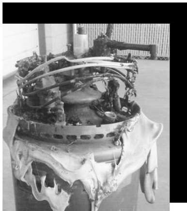
Liquid Oxygen Reservoir — After a Fire
